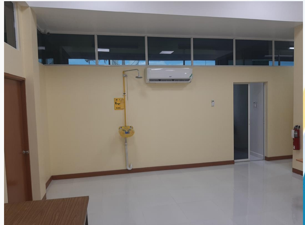
Common Area with emergency Shower
